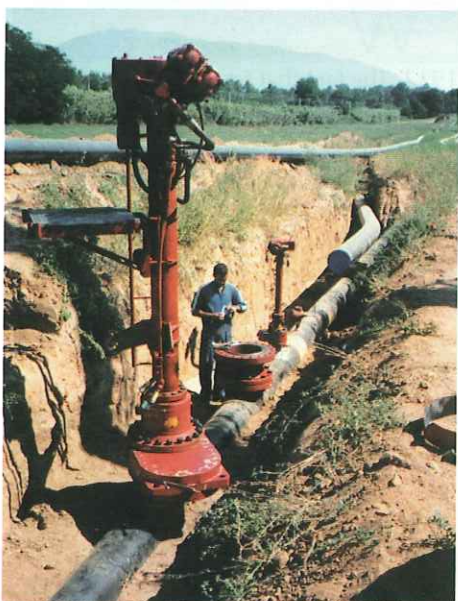
Preparation of an operation to incorporate a 20-inch, variant in the fluid transport pipe, without stopping the flow at any time.
