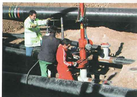
Double sealing work on a piping rack for petrol-chemical fluids and gas. Fluids are continually flowing through the pipes.
